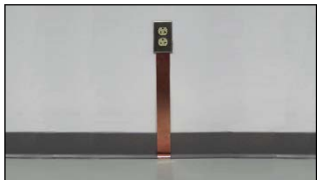
Figure 5. ESD Floor Ground Strip
